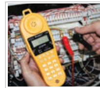
Telephone line testing
