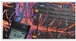
Fiber optic power test
