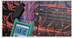
Fiber optic power test
